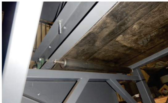
Fig. 6. Access to the catching area between the support roller and the belt and between the belt and the conveyor frame
