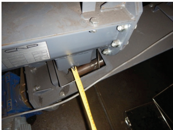
Fig. 10. Access to the entanglement and crushing zone in the screw conveyor
